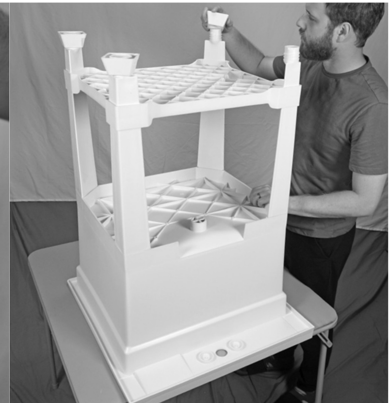
6 Take a minute to inspect all fittings and secure as needed. Position the sink so the drain and faucet can be connected next.
